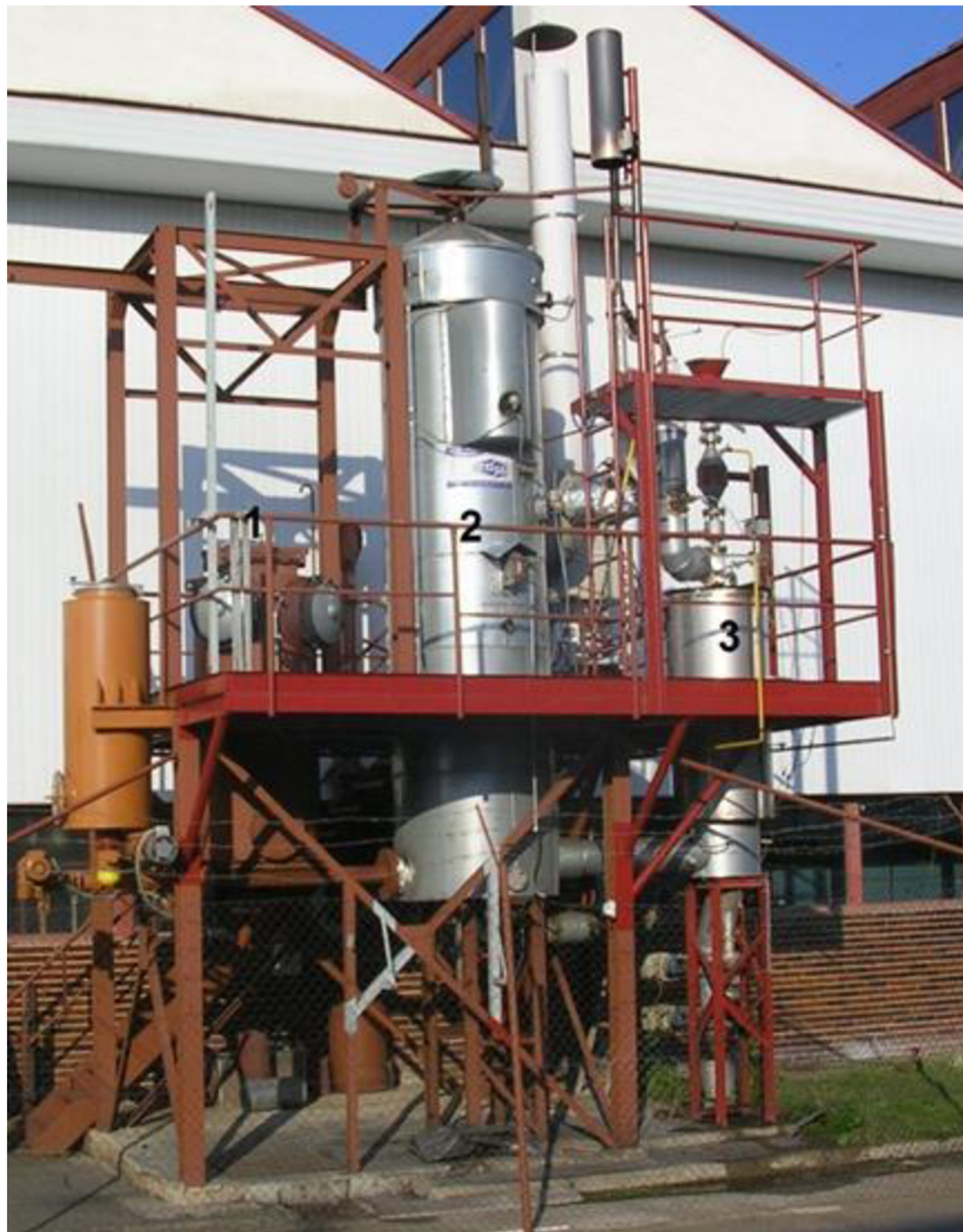
Figure 13 : Atmospheric fluidized bed gasifier Biofluid 100
