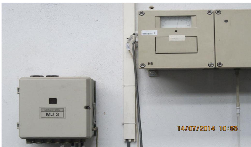
Figure 18 :Connecting the measuring units MJ3 (used only for measurement hydrogen content in the produced gas -online measurement)
