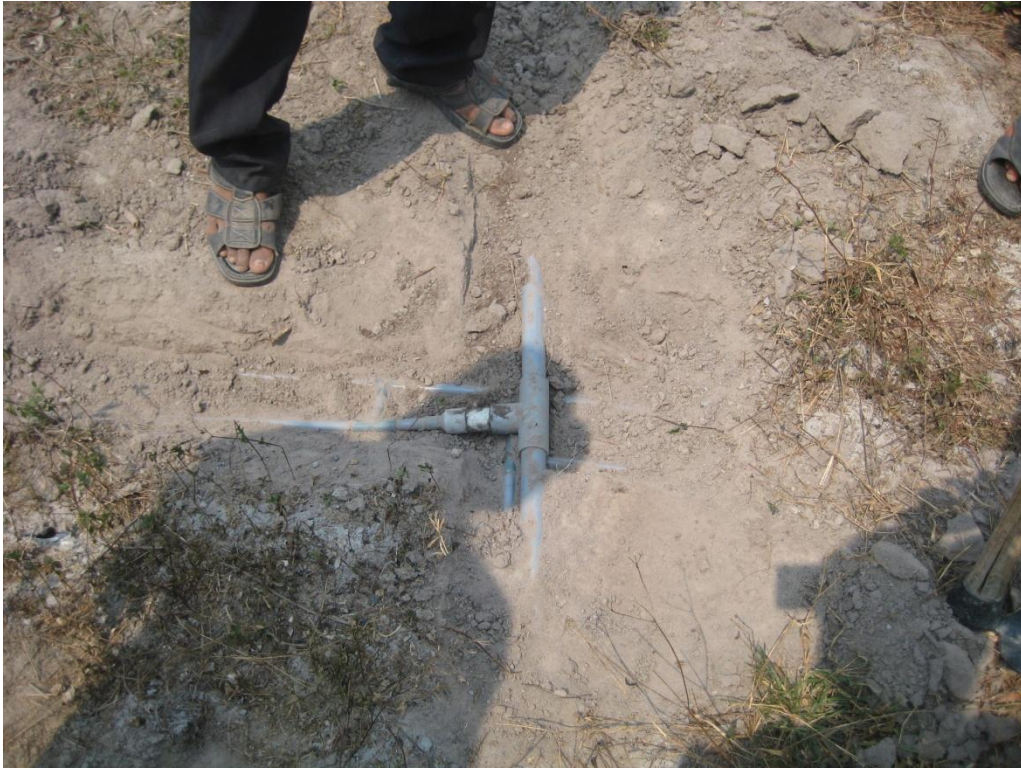
Figure 31: The underground PVC pipe mesh of exited irrigation system
