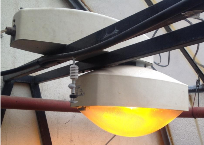
Figure 3: Czechoslovakian street lamp fixture with cover (Photo: Author).
