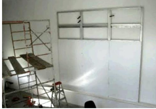
Figure 3.15: Aluminum structural framework for a geotextile living wall. It is in the second phase of construction and partially covered by white rigid PVC sheets (Source: Irwin 2012).
