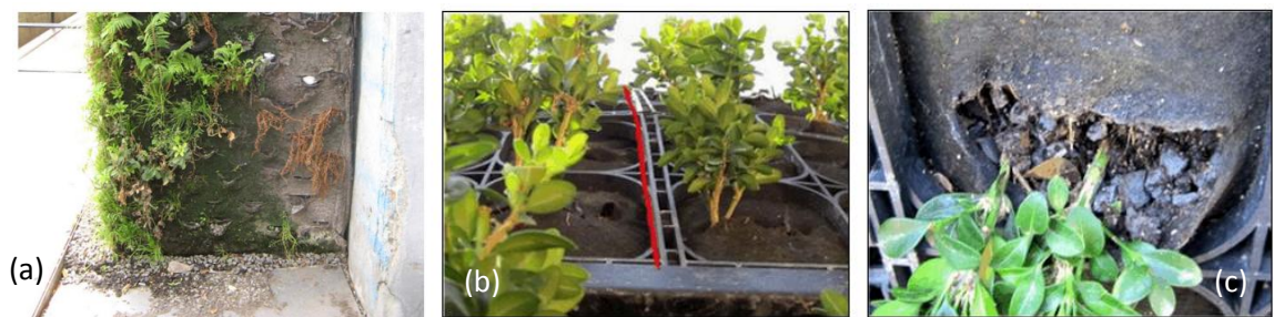
Figure 3.14: (a) Wall failing due to poor design and inadequate maintenance (Source: Perini et al. 2011). (b) and (c) Structure damaged by weight of the wall, red line shows wall bend (Source: Irwin 2012).
