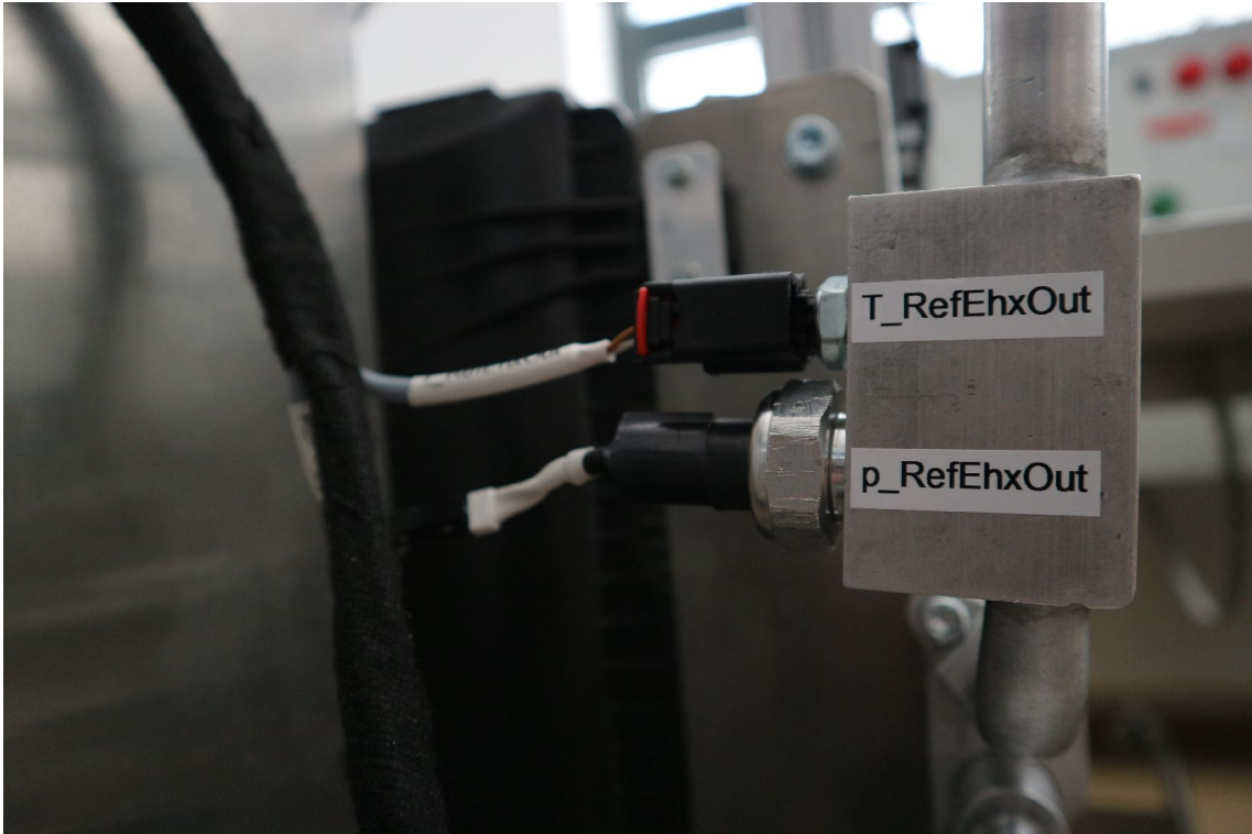
Fig. B.9: Refrigerant temperature and pressure sensors
