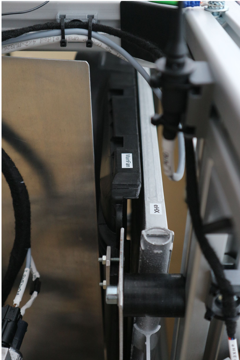
Fig. B.15: External heat exchanger (eHX) and Main Fan
