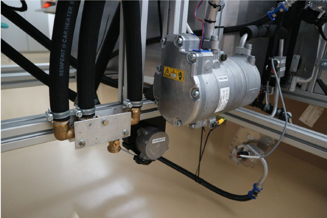
Fig. B.5: HV compressor and coolant pump
