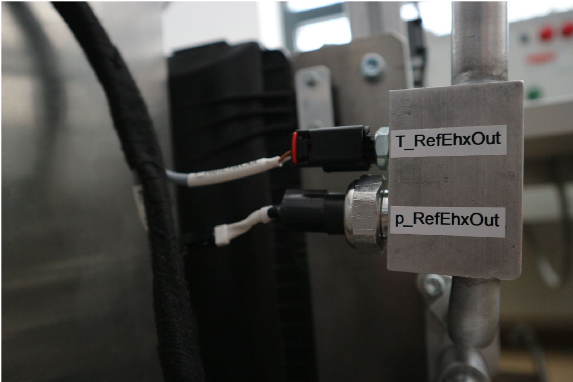
Fig. B.9: Refrigerant temperature and pressure sensors
