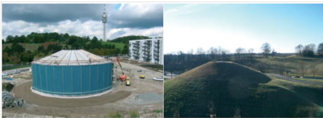
Fig. 10.5 Large Hot water storage (construction and final state) [33]
