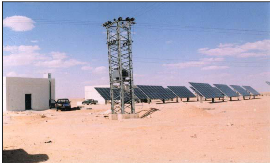
Fig. 4.5 Wade Marsite PV Central Plant [11]
