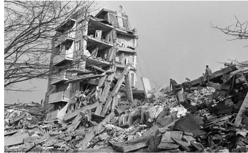
Figure 25: Residential building after disaster Source: newizv.ru
