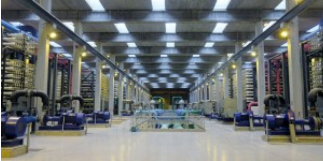
Figure 18: Reverse Osmosis (Blending Technologies 2016)
