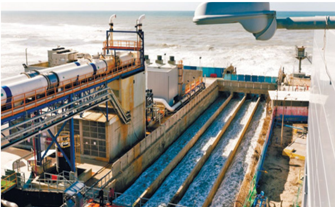
Figure 20: Desalination plant in Israel (Zafir Rinat 2019)
