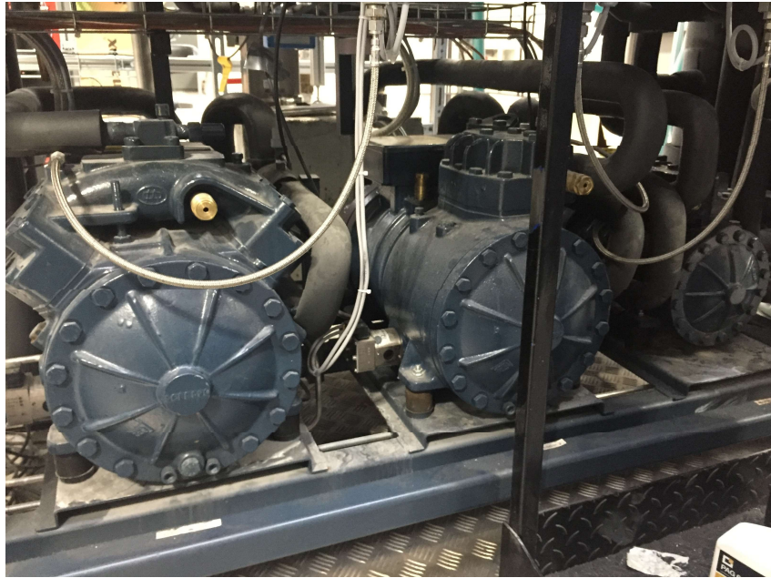
Figure 4.2 R744 piston-type compressors pack. Base-load compressor (Dorin CD1400H) at the left and parallel compressors (Dorin CD1000H and Dorin CD380H) at the right.
