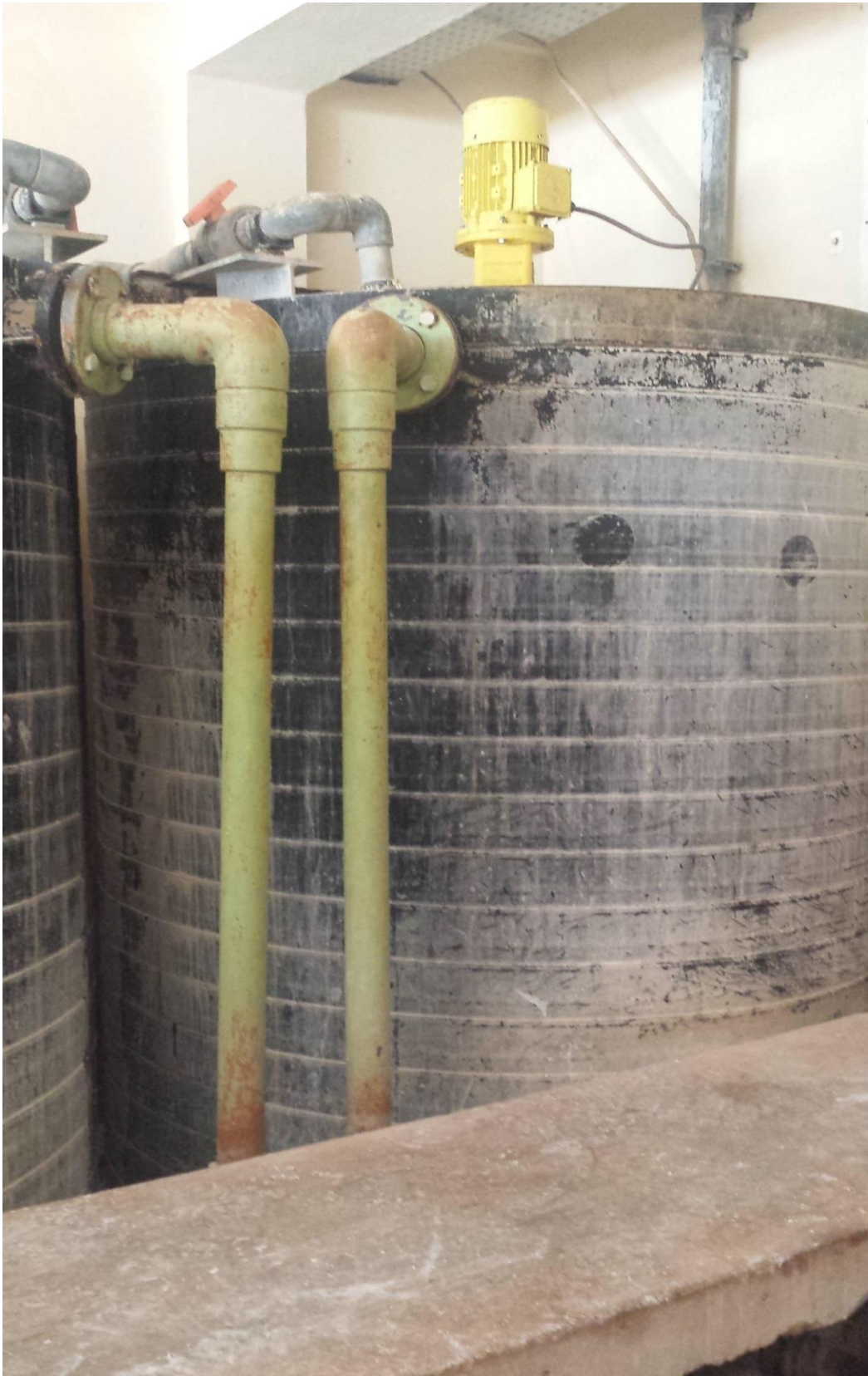
Figure 6: Ca (ClO) 2 tanks
