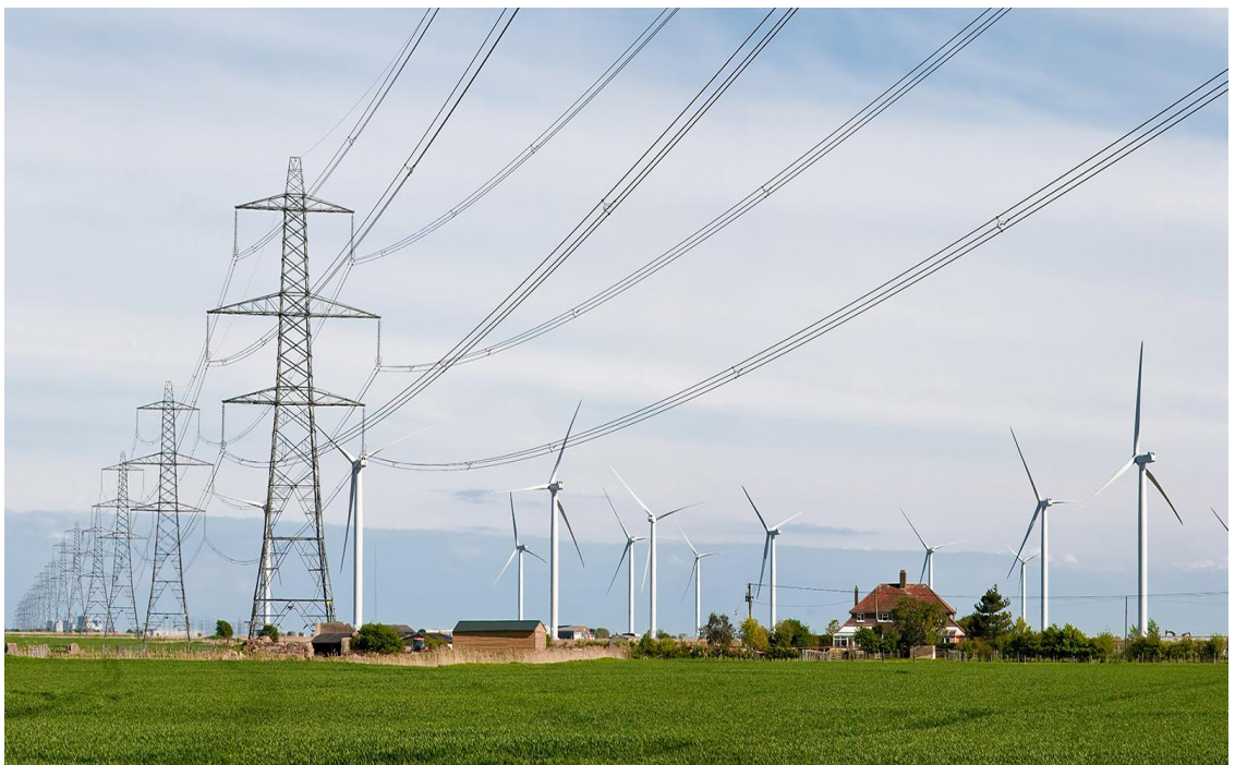
Figure 3.1: Electricity Transmission Line
