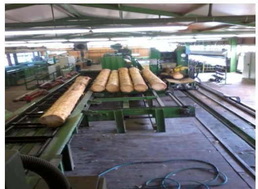
Figure no. 12: Feeding longitudinal conveyor belt
