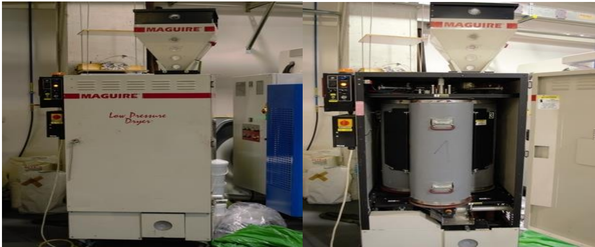
Fig. 12: Low pressure dryer
