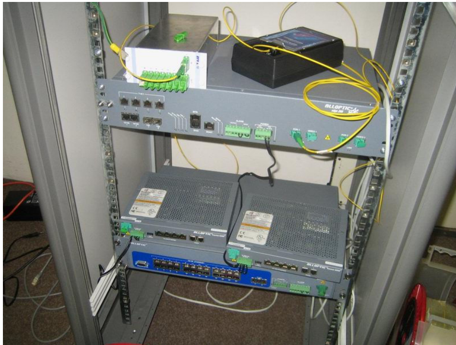
Fig. 41: PON network devices and 1:8 passive splitter
