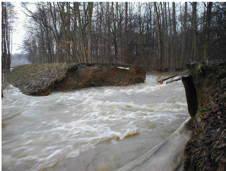
Fig. 6.7 Fourth phase: dike collapse
