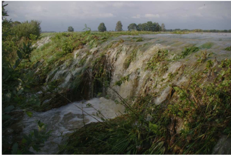
Fig. 6.6 Third phase: erosion - no collapse
