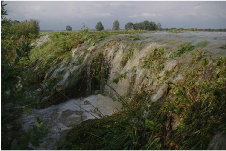
Fig. 6.6 Third phase: erosion - no collapse
