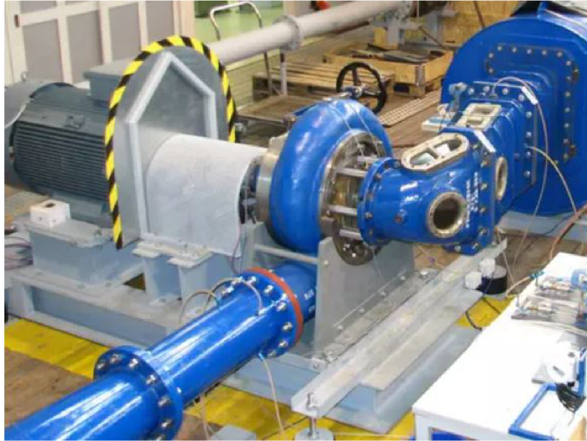
Figure 3: Installation site of PAT [3]
