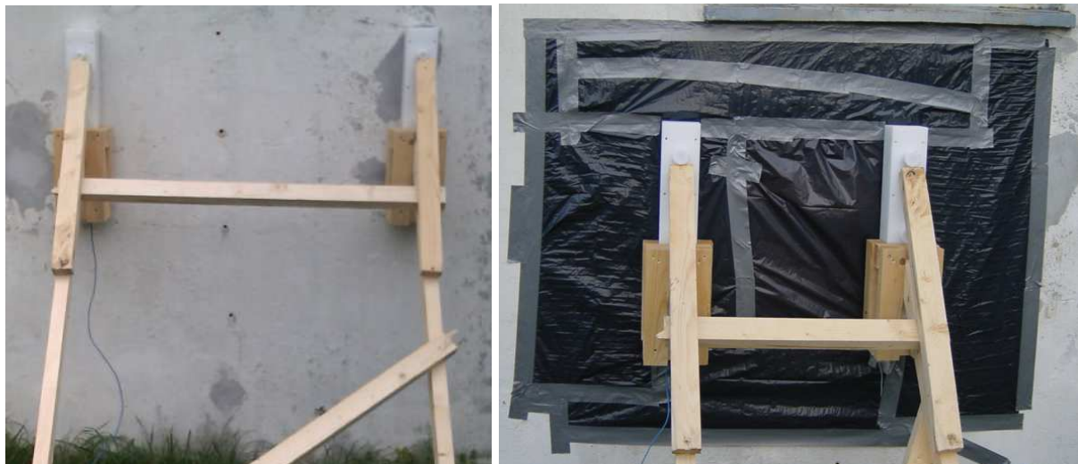
Fig. 62 The placement of the electrode units on the wall, wooden construction and the area of the wrapping in the second stage.
