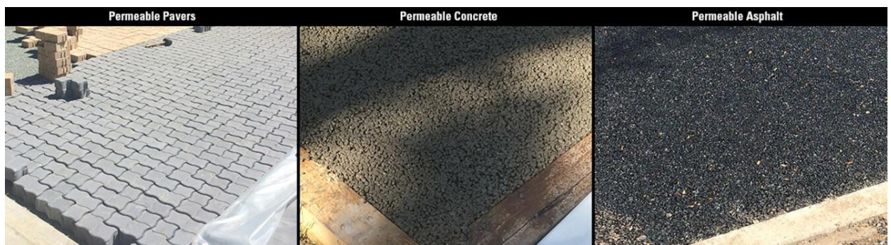
Figure 4 Installations of the three test pavement types: permeable pavers, permeable concrete, and permeable asphalt ( Upper Midwest Water Science Center , 2019)
