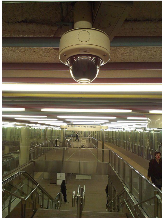
Figure 13 Dome camera in a rail station
