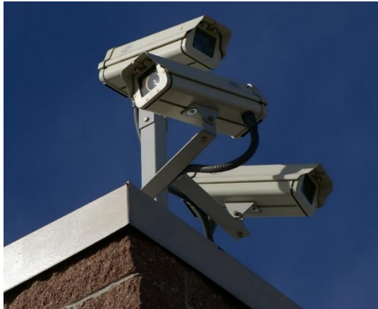
Figure 11 Three bullet cameras on the corner of a building
