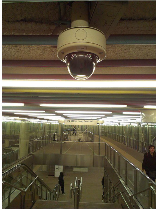
Figure 13 Dome camera in a rail station
