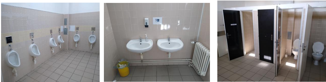
Figure 31 Washbasins and urinals in the school building.
