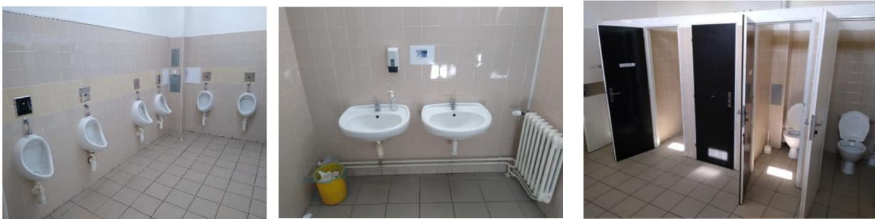
Figure 31 Washbasins and urinals in the school building.
