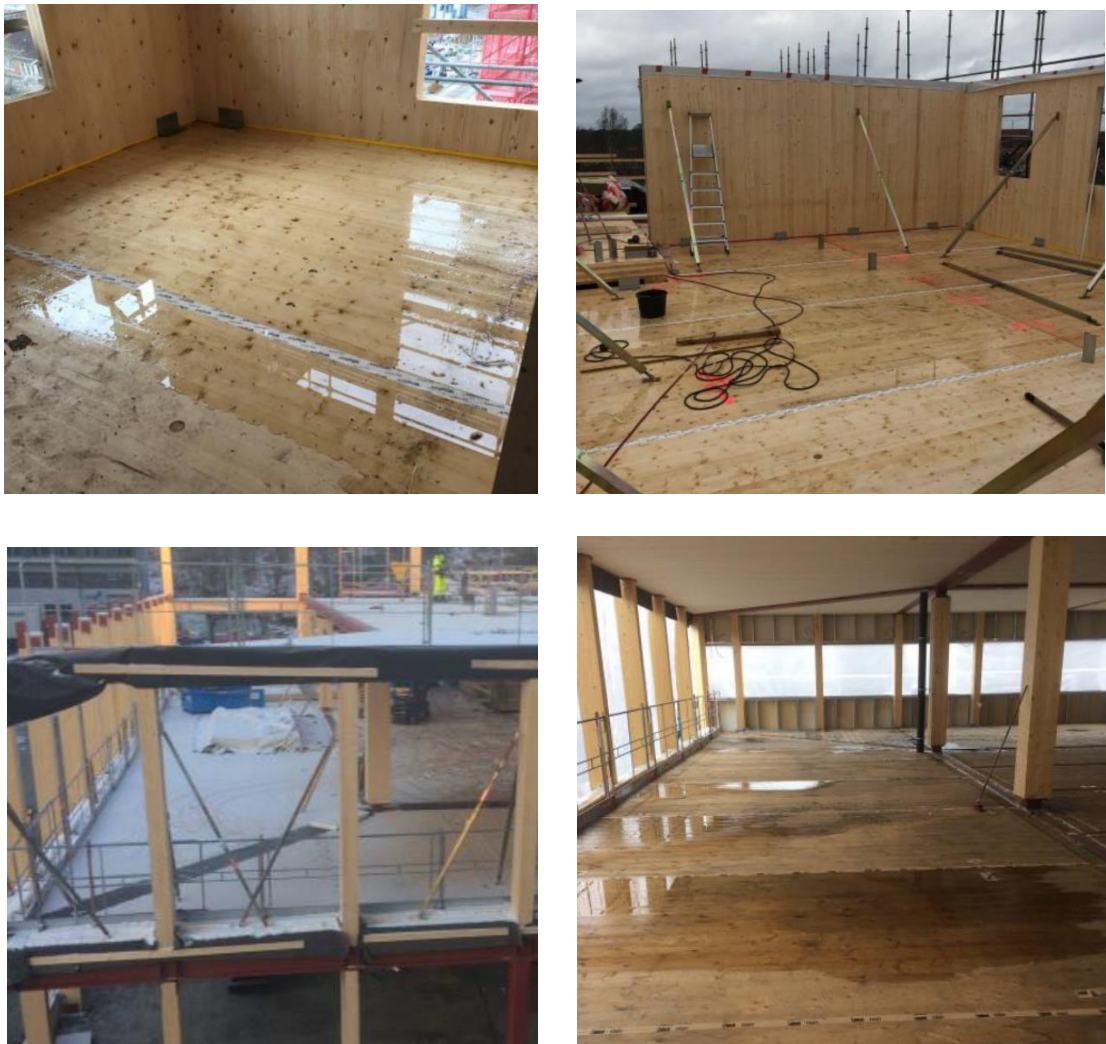
Figure 27 - CLT panel ceiling exposed to pooled water (Olsson, 2020)
