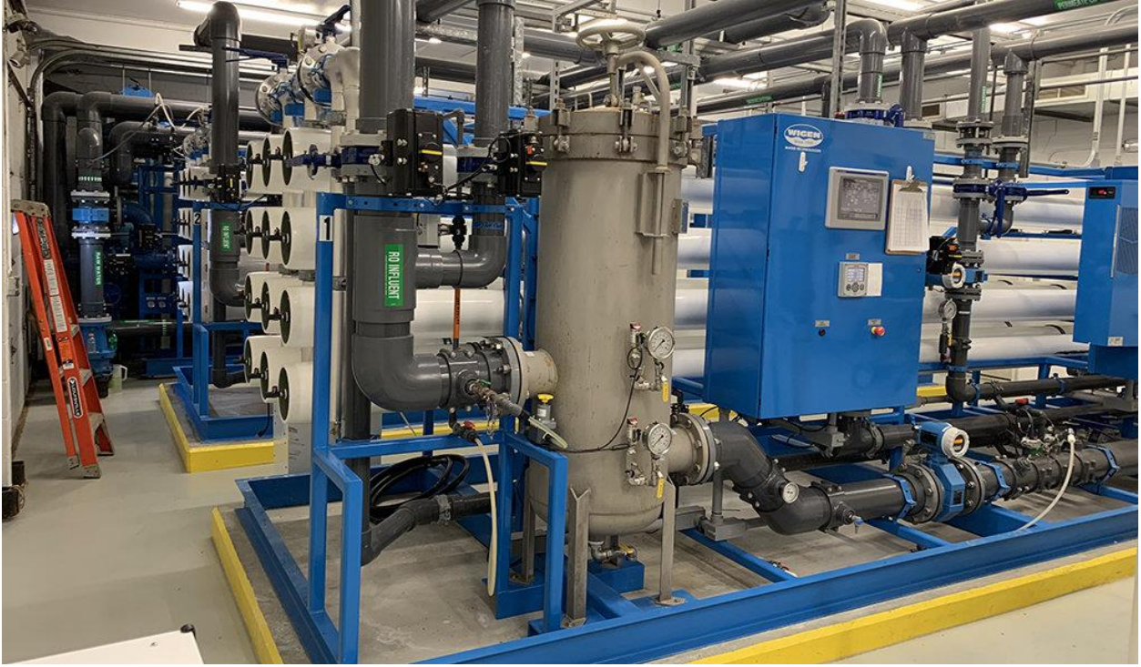
Figure 28 Reverse osmosis technology
