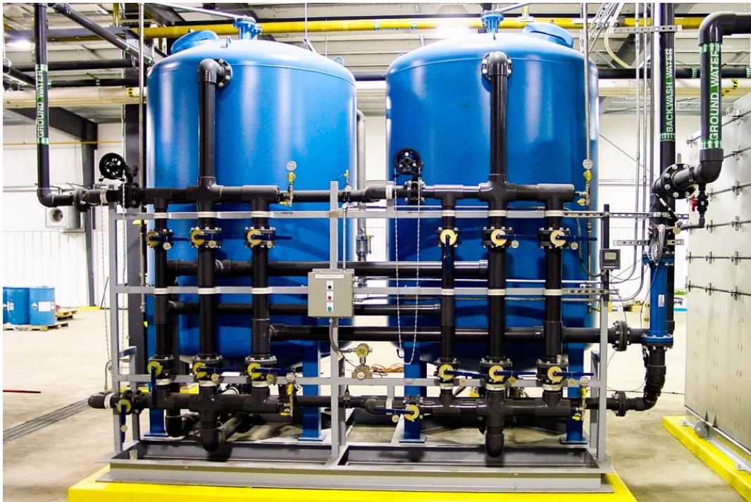
Figure 22 Carbon filtration system
