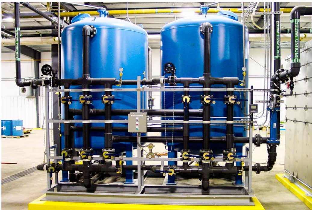
Figure 22 Carbon filtration system
