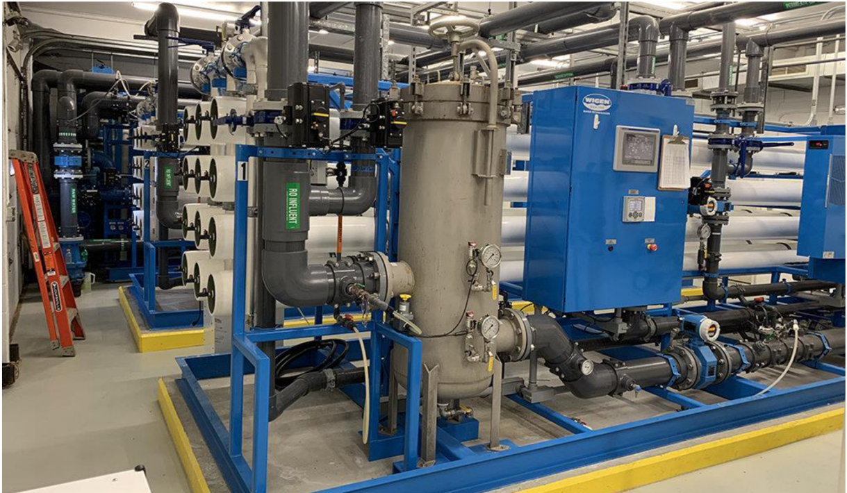
Figure 28 Reverse osmosis technology
