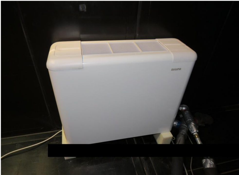
Fig. 5 Overall view of the fancoil installed in calorimeter chamber
