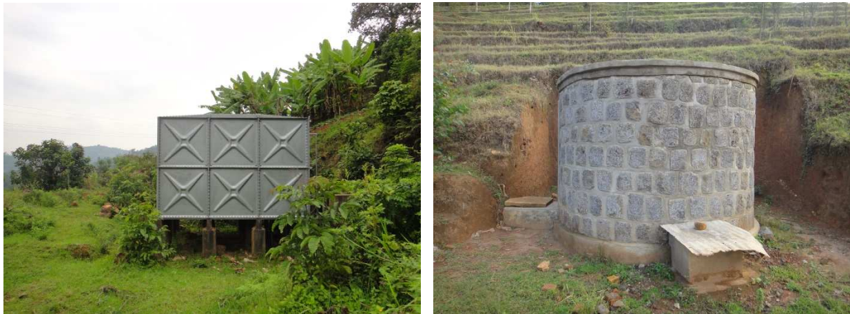
Figure 6: Main storage tank (left) and tank Future for Kids (right) (own pictures, 2014)
