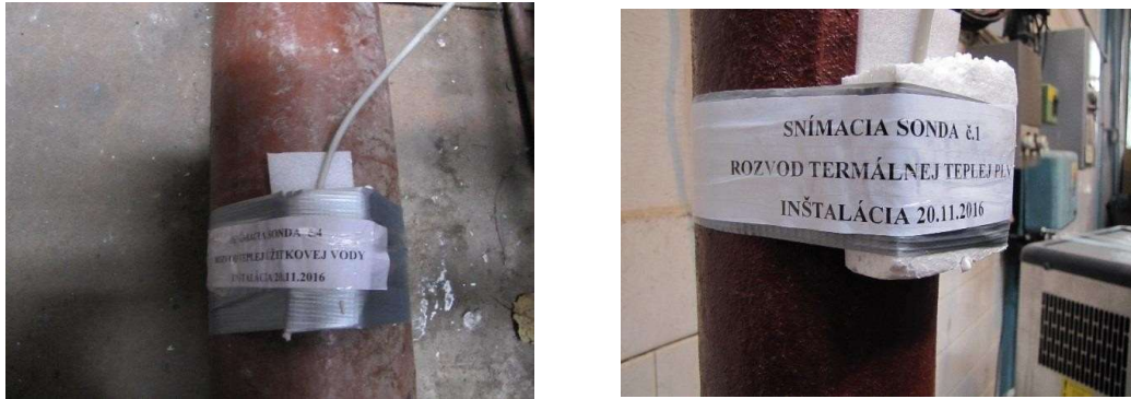
Picture 4.21. Left: Temperature sensor at hot service water (yellow pipeline), Right: Temperature sensor at hot natural healing water (red pipeline) [9]
